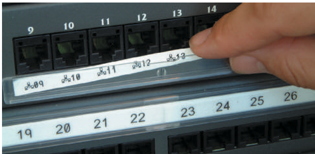
Punch block & patch panel labels
