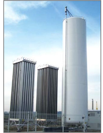
AC SCS-LNG Line Bulk Tanks
